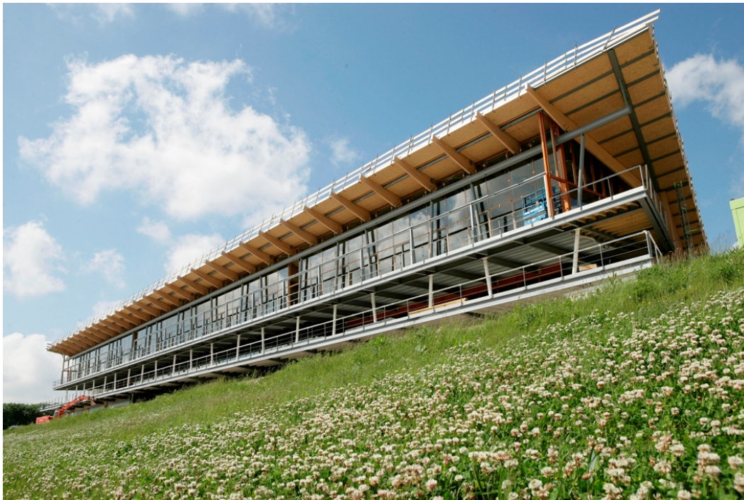
Figure 6. Office building under construction on top of a landfill.
