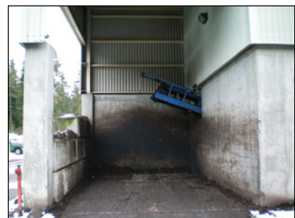
Photo 9-4: A temporary storage area can decouple systems in the facility and provide operators with some flexibility to schedule daily tasks © CH2M HILL
