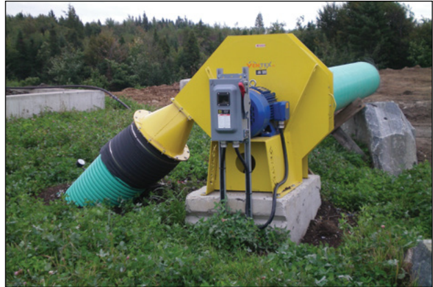
Photo 8-3: Aeration fans used at composting facilities normally require three-phase power supply © CH2M HILL
