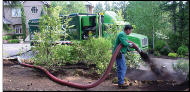
Photo 17-1: Blower trucks are commonly used to place or spread compost for erosion control applications © Rexius Forest By-Products Inc.
