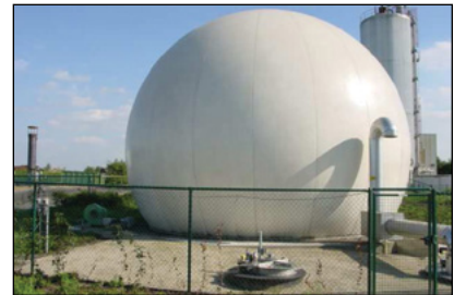
Photo 4-1: Biogas storage tank © Organic Waste Systems Inc.
