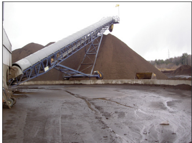
Photo 11-17: Radial stacking conveyor © Scott Gamble
