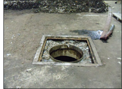
Photo 10-8: Underground sumps and tanks are commonly used to collect and store high-strength leachate © CH2M HILL
