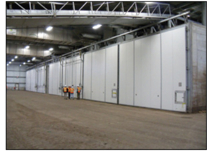
Photo 5-17: Enclosed tunnel composting system © CH2M HILL
