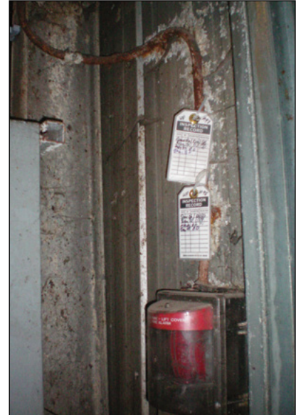
Photo 9-3: Fire detection and alarm systems inside organic processing facilities are particularly susceptible to damage from corrosion © CH2M HILL
