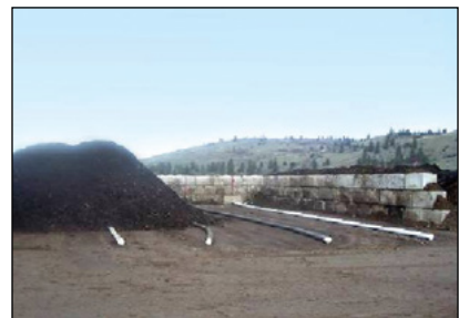
Photo 5-13: Typical ASP system with aboveground piping; block walls separate batches to better utilize available space © CH2M HILL
