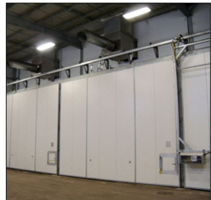
Photo 5-18: Closeup of tunnel door system © CH2M HILL
