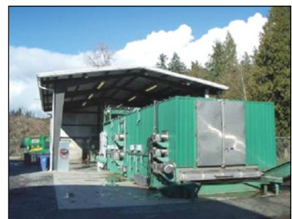
Photo 5-23: Agitated container composting system installed at a university campus © CH2M HILL
