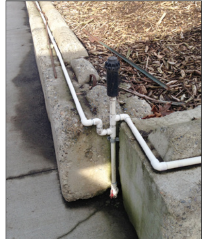
Photo 14-7: Water can be added to biofilter media using sprinklers, but care must be taken not to overwater the biofilter media © CH2M HILL
